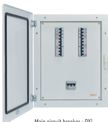
Main circuit breaker : DX 3
