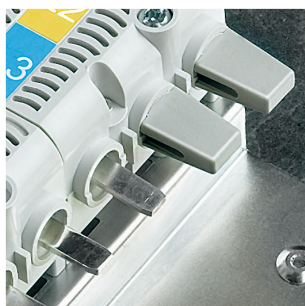
Insulated terminal shields on outgoing terminals that are not in use (provided with the distribution board).
