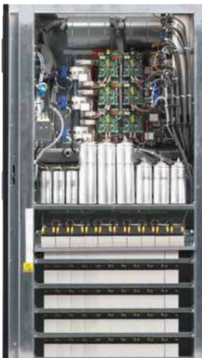
INTERNAL BATTERY FIXTURES
