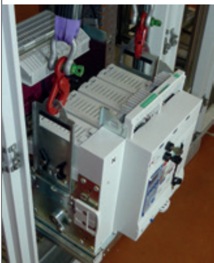
Installing a draw-out DMX 3 in its base
