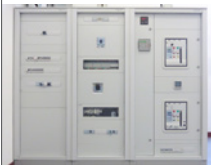
4000 A assembly with DMX 3 supply inverter at the supply end
