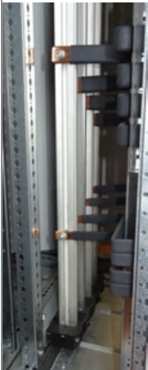
Busbar installed in cable sleeve.
